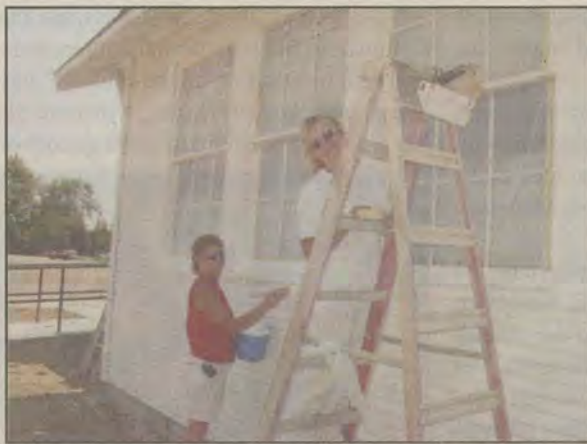
Kathie Veenstra and Camy Burns of Hamilton & Spear, the contractor hired by Walt Morrow Construction for the City of Meridian.
