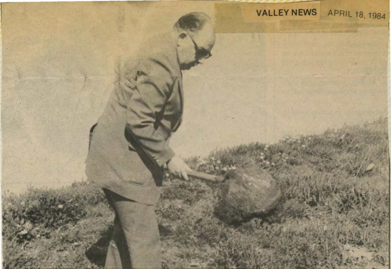
Meridian Library District chairman Jack Riddlemoser turns the first shovel-full of earth, kicking off a $50,000 expansion project.
